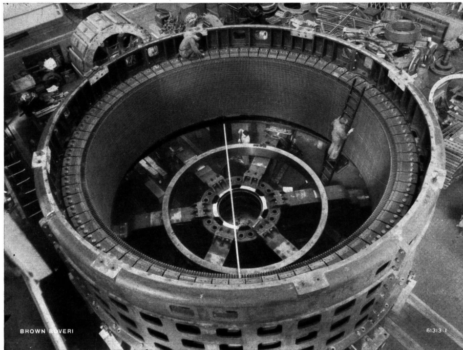
Fig. 17. — A crane driver's view of the stator and lower bearing spider of the 25,000 kVA single-phase generator for the Rupperswil-Auenstein power station during erection.
