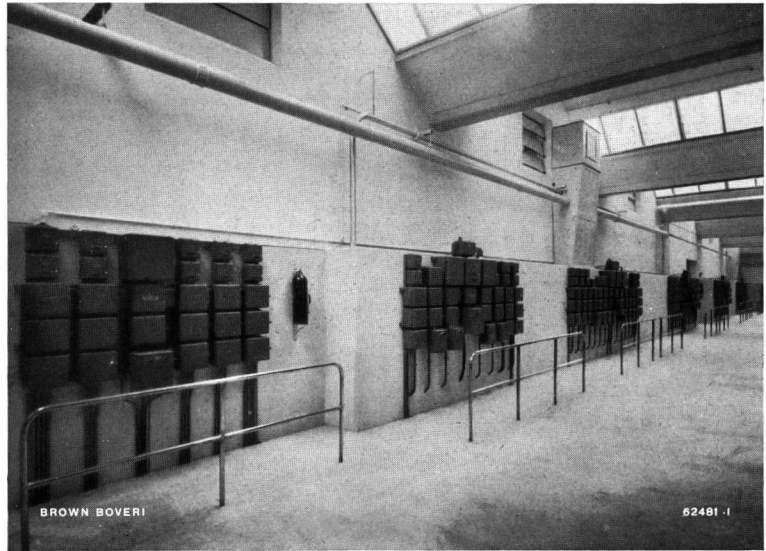
Fig. 65. — Banks of switchgear for 86 individual drives in the blowing room of a cotton spinning mill.
