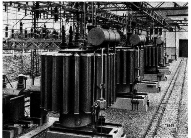
Fig. 1. — The Seebach Substation of the Swiss Federal Railways.
