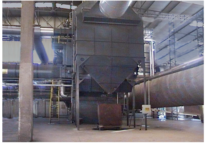
The upgrade minimized the need for intervention by the operators and incorporated safety interlocks into the process.
