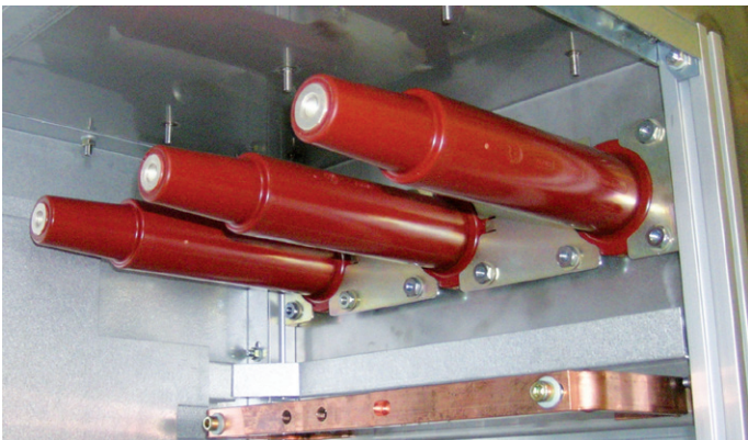
Fig. 7.5.1: View into the cable termination area with outer cones termination type C in air, without cable connectors (during assembly at the works, without the cable termination compartment)
