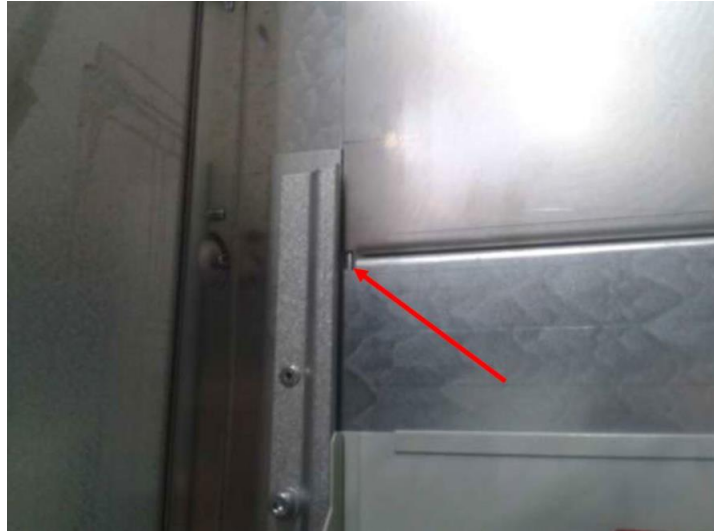
Figure 3 Opening between circuit breaker and busbar compartment
