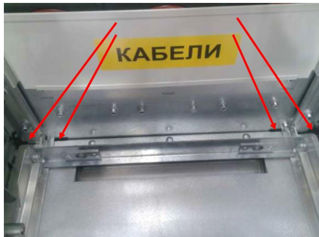
Figure 2 Openings bigger than 2,5mm between circuit breaker and cable compartment
