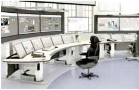
System 800xA control room
