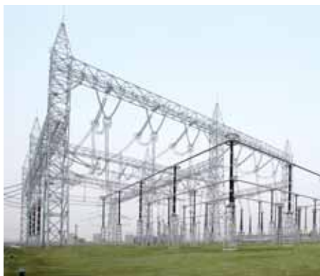
Strengthening Bangladesh's power network
