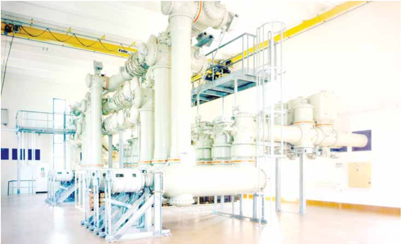
380 kilovolt gas insulated substation to facilitate power reliability
