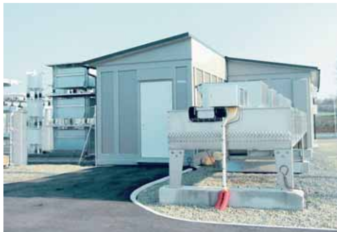
Outdoor substation module for mainline railway
