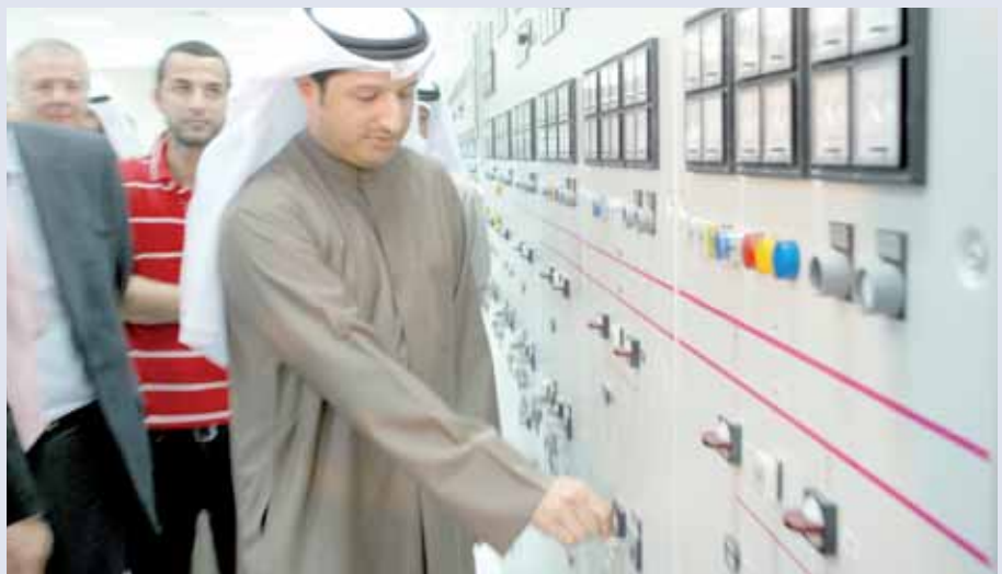
His Excellency the Minister for Electricity and Water for Kuwait Dr Bader Al-Sherean inaugurating the Sulaibiya substation
