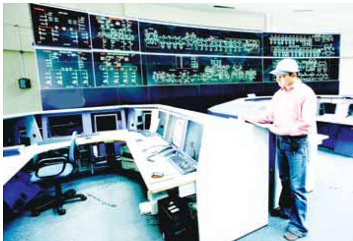
SCADA control room for a metro rail power system
