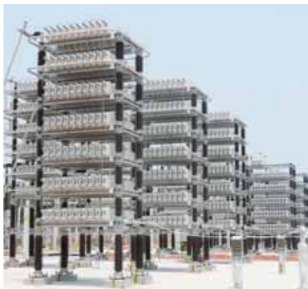
HVDC Light solution to boost power capacity
