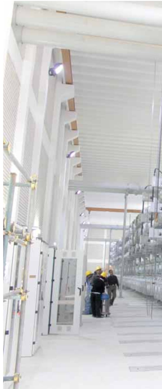
400 kV gas insulated switchgear room at Sulaibiya substation
