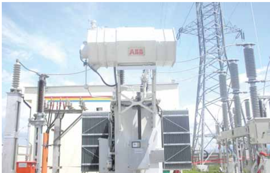
110/20 kV Harman transformer substation
