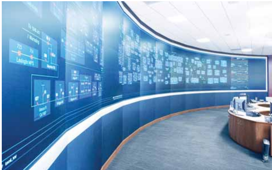
SCADA control room enables real-time monitoring of OIL assets
