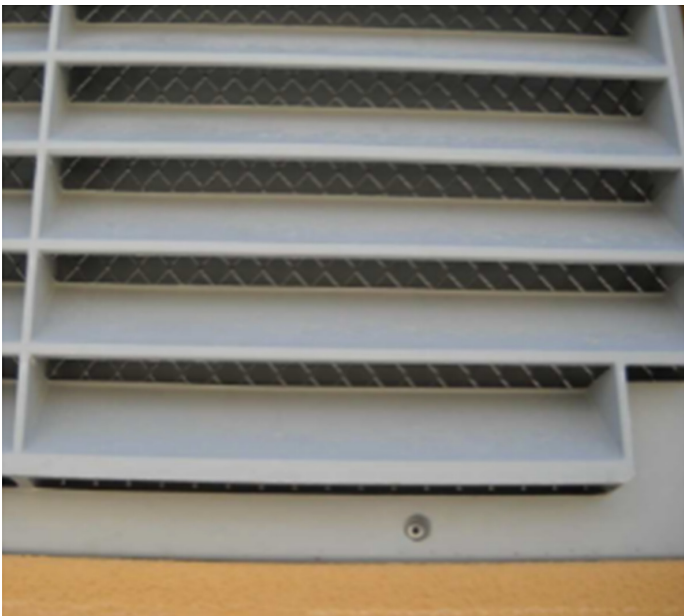
Fig. 8 : example of a ventilation opening with grating
