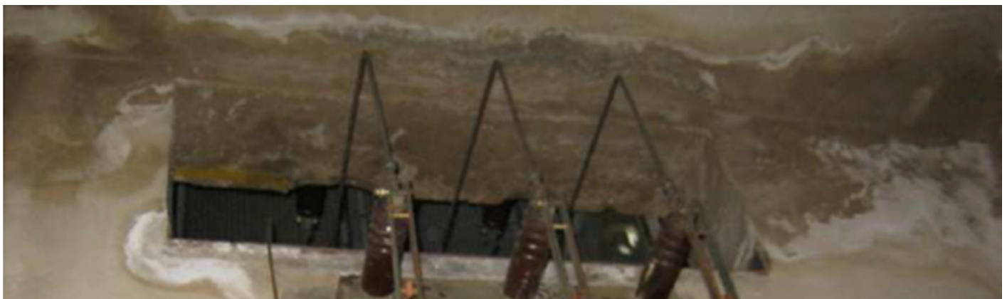
Figure 2: example of a substation where water is infiltrating through the ceiling
