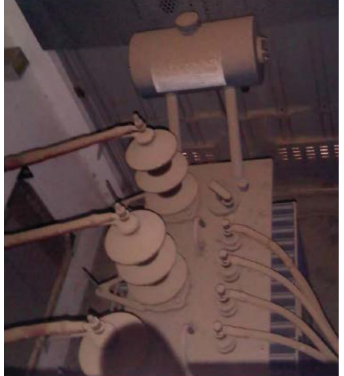
Fig. 5 : example of a substation where thick dust and other pollutants have built up on the apparatus
