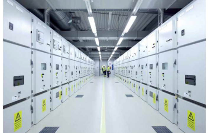
Fig. 10 : example of an MV substation with UniGear switchgear
