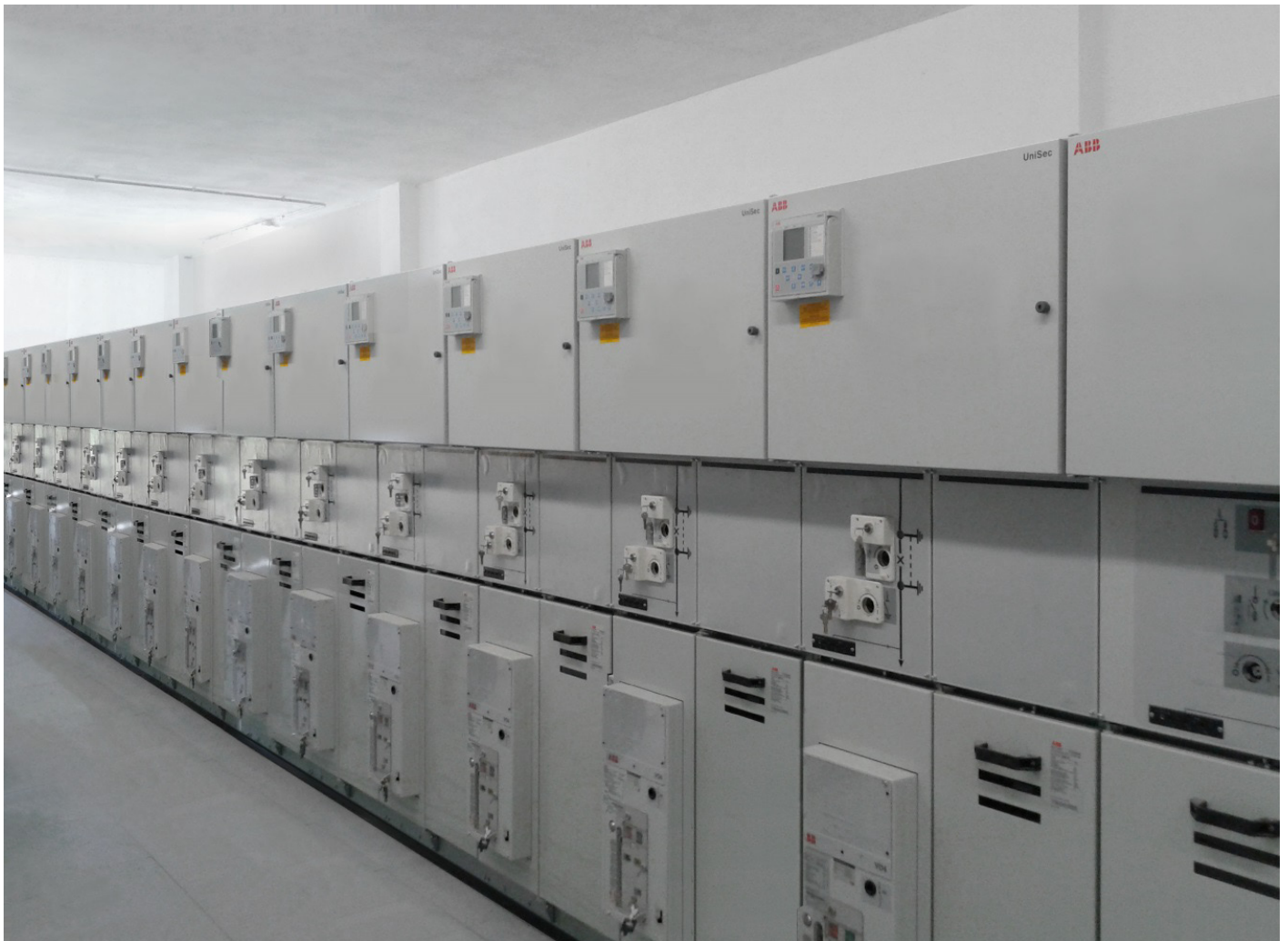
Fig. 1 Example of a medium voltage substation with UniSec switchgear
