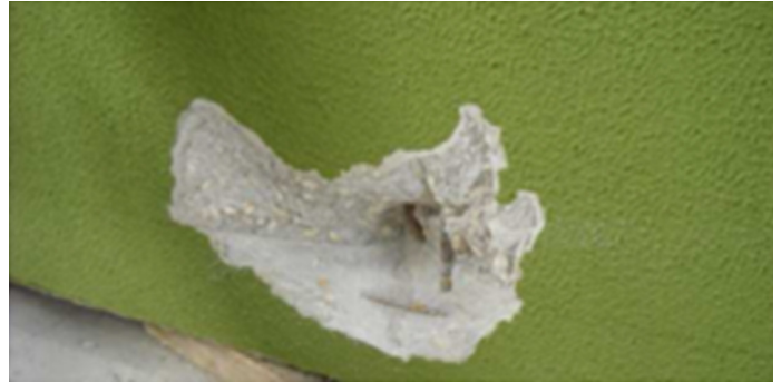
Figure 3: example of external damage through which water can seep
