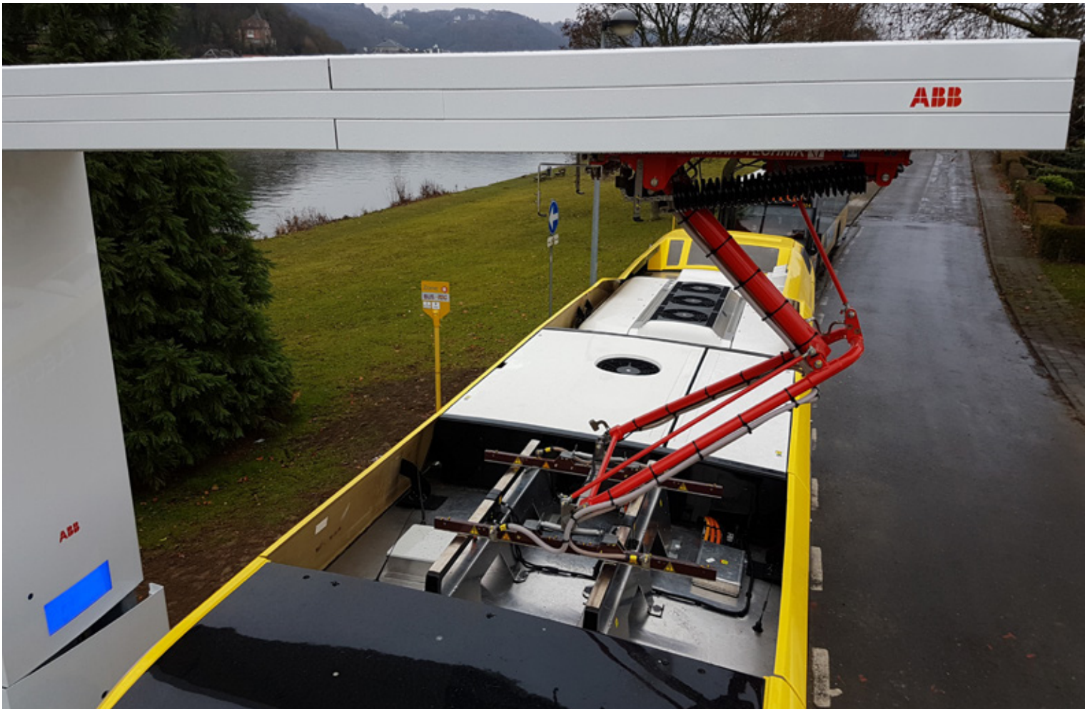
— A close-up view of an overhead pantograph to eBus connection using the OppCharge standard
