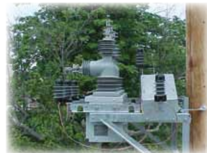
Surge arresters and potential transformers are easily adaptable with our brackets on the mounting frame.
