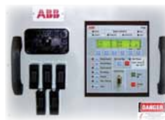
Substation rack mount
