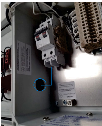
Figure 3-3: Incoming Power (Customer Provided)
