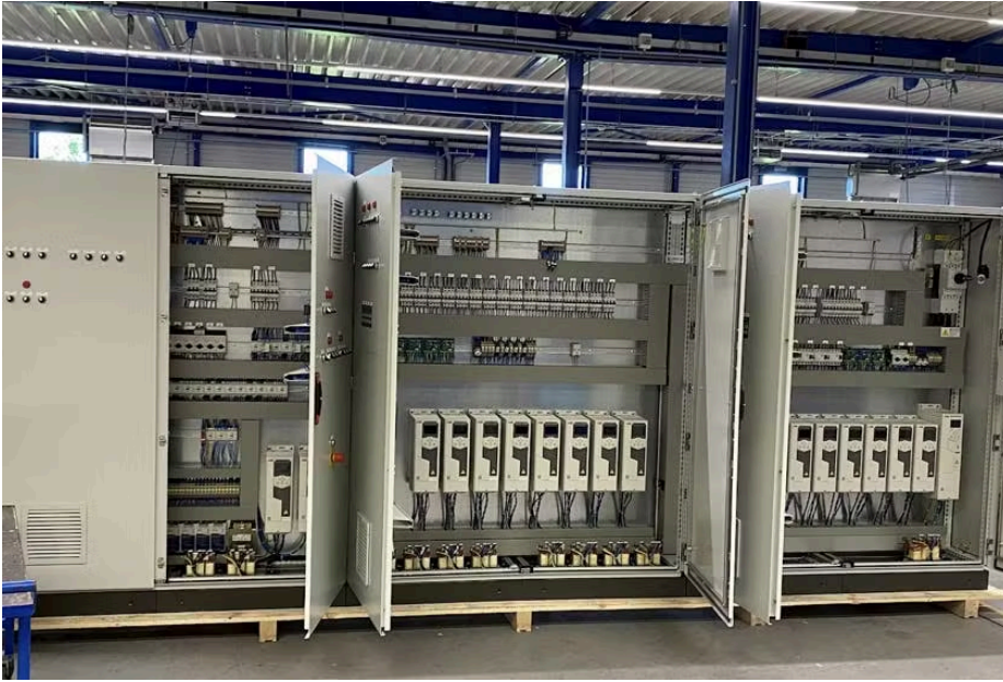
ABB drives control ventilation, egg control and material conveying. Source: ABB
