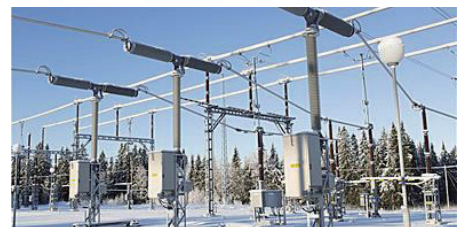
State Grid Jinhua Smart Substation
