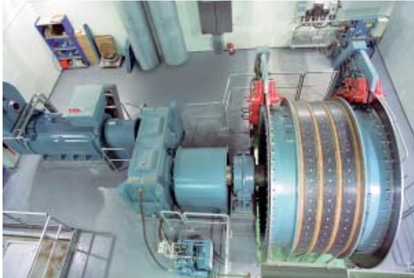
Production hoist with 1,600 kW induction motor
