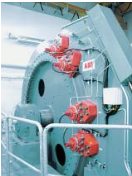
Disc brake system for the production hoist
