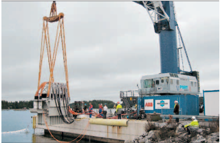
3 A 16.5 MVA transformer being submerged for a heat run and system testing at Vaasa harbor, Finland. The three 22 kV penetrators and two low voltage signal connectors are visible
