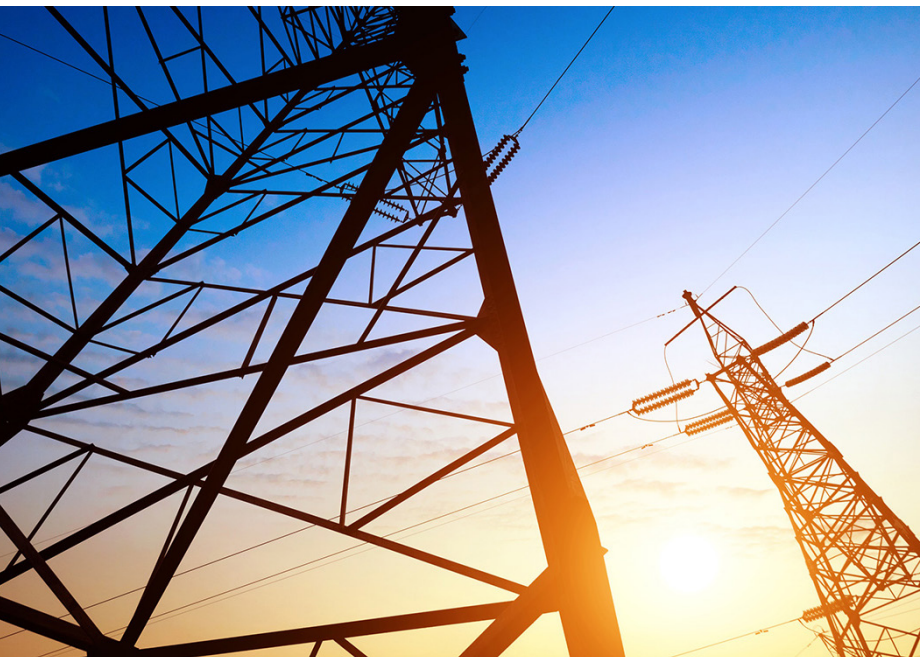
01 A typical substation electric tower
