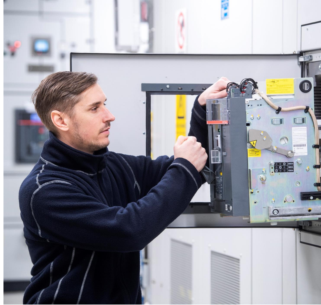
AstraZeneca pharmaceutical manufacturing, Sweden Solution: Retrofitting electrical assets
