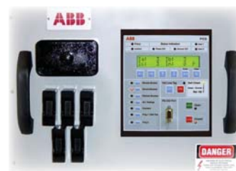
Substation rack mount
