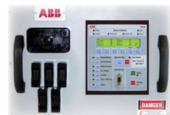
Substation rack mount
