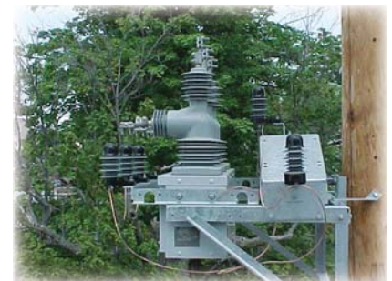
Surge arresters and potential transformers are easily adaptable with our brackets on the mounting frame.
