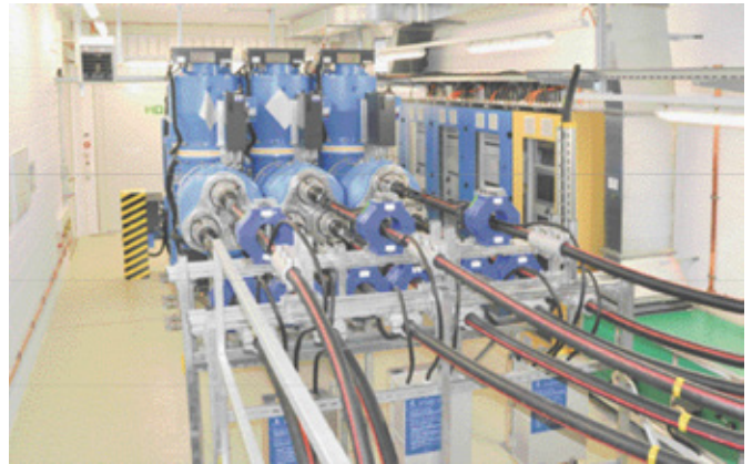
San Bernardino substation
