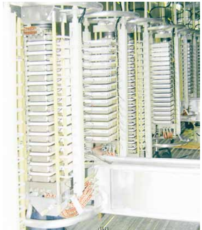
SVC Light® valve assembly.
