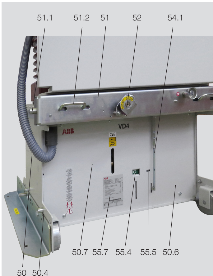
Figure 6/3: Circuit-breaker, type VD4, on withdrawable part. Control area
