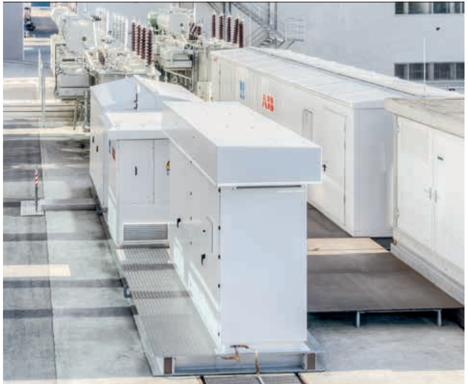
5 1 MW/15 min EssPro Grid BESS at EKZ in Dietikon, Switzerland
