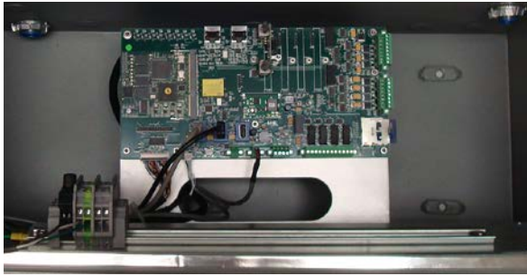
Figure 4.2. Inside the Master Controller
