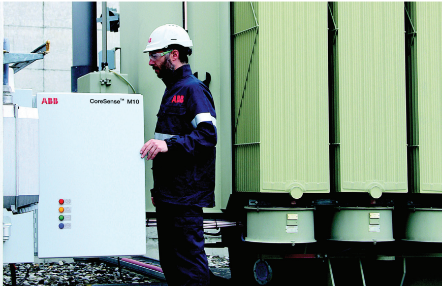
01 CoreSense™ M10 installed on a transformer at CERN, the European Organization for Nuclear Research in Switzerland
