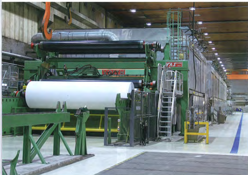
PM 2 is now running with new drives
