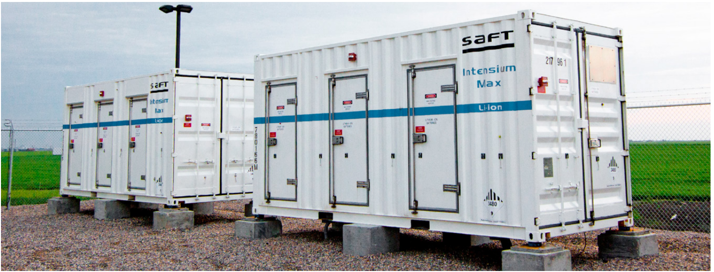
SAFT battery containers at the CFN wind generation site. ABB's compact EssPro PCS Power Conversion System package is housed inside. Images courtesy of Saskatchewan Research Council.
