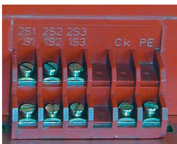
Fig. 2. 1 Secondary terminal box (3 secondaries and voltage indicator)
