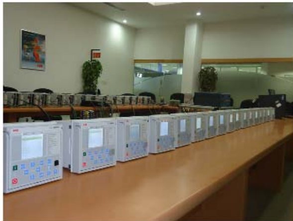
Fig. 12 Factory acceptance test set-up
