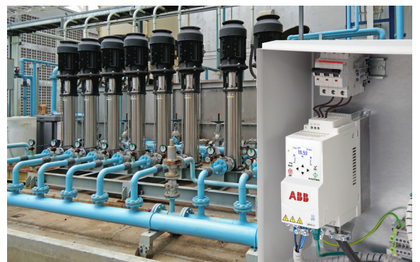
There are a variety of different inputs and control schemes that may be applied to the drive being used on pumping applications.
