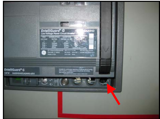
Fig. 1 Remote Racking Operator mounting Port.
