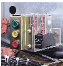
SF6 control device with 3 LEDs.
