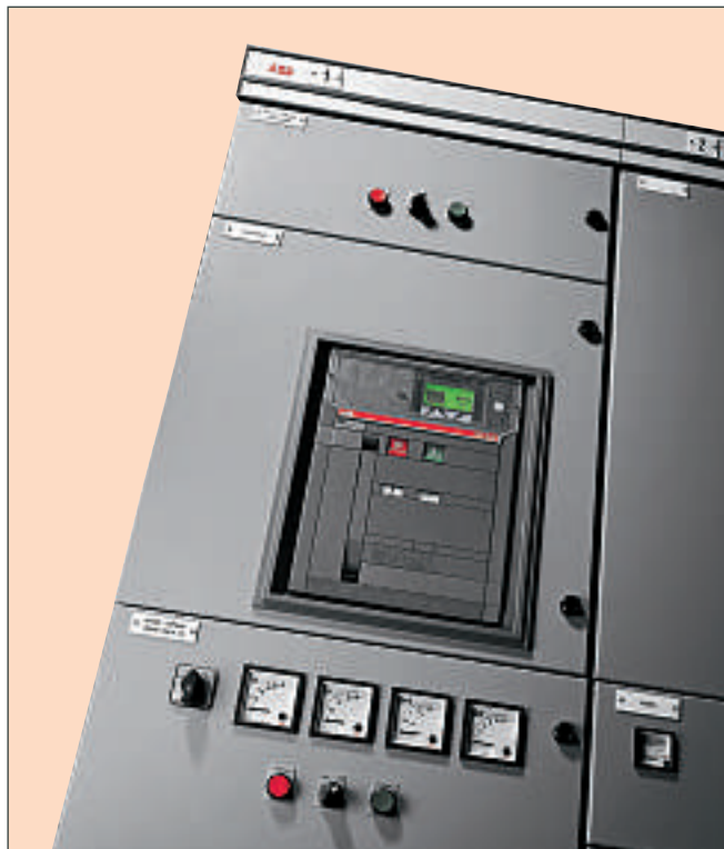
2 A typical circuit-breaker installation in a switchboard – occasionally uncomfortable for users.
