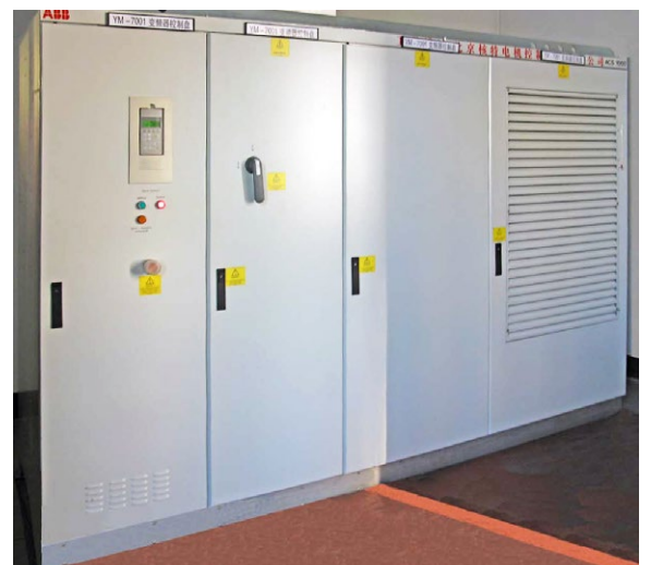
ACS1000 variable speed drive controlling the mixer at the Daqing Petrochemical Plastic Factory in China.
