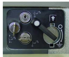
Interlocks on earthing switch operating mechanism
