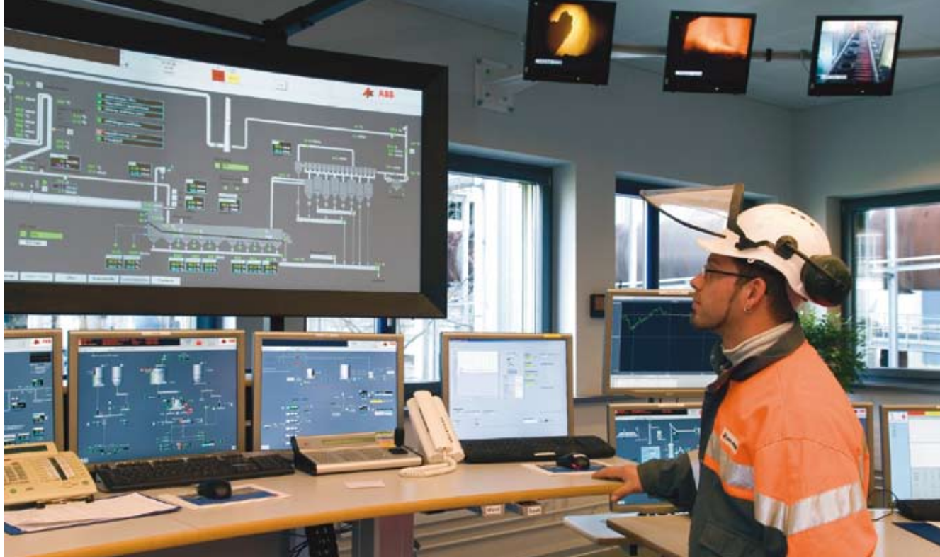
Figure 8. ABB 800xA Control System, cpmPlus Expert Optimizer and Knowledge Manager are installed at the Jura cement plant, Switzerland.
