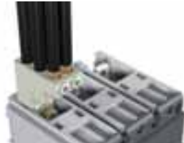
Multi-cable terminals with cables
