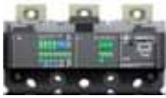
Loose trip unit
