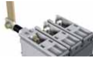
R terminal with vertical busbar
