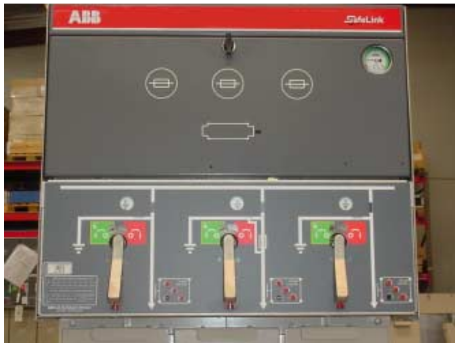
Front of SafeLink unit showing the mimic diagram and switches in (from left to right) the off, on, and earth positions.
