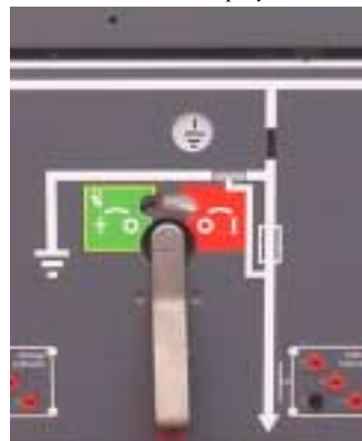
Front of SafeLink unit showing the mimic diagram for the switch-fuse following a fuse blow event. Note the word 'RESET' and the red fuse blown indicator are displayed.
