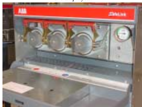
Fuse door open and fuse canisters available.
