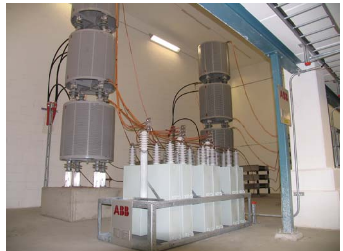
Figure 5. Filter unit installed at Malmberget processing plant
