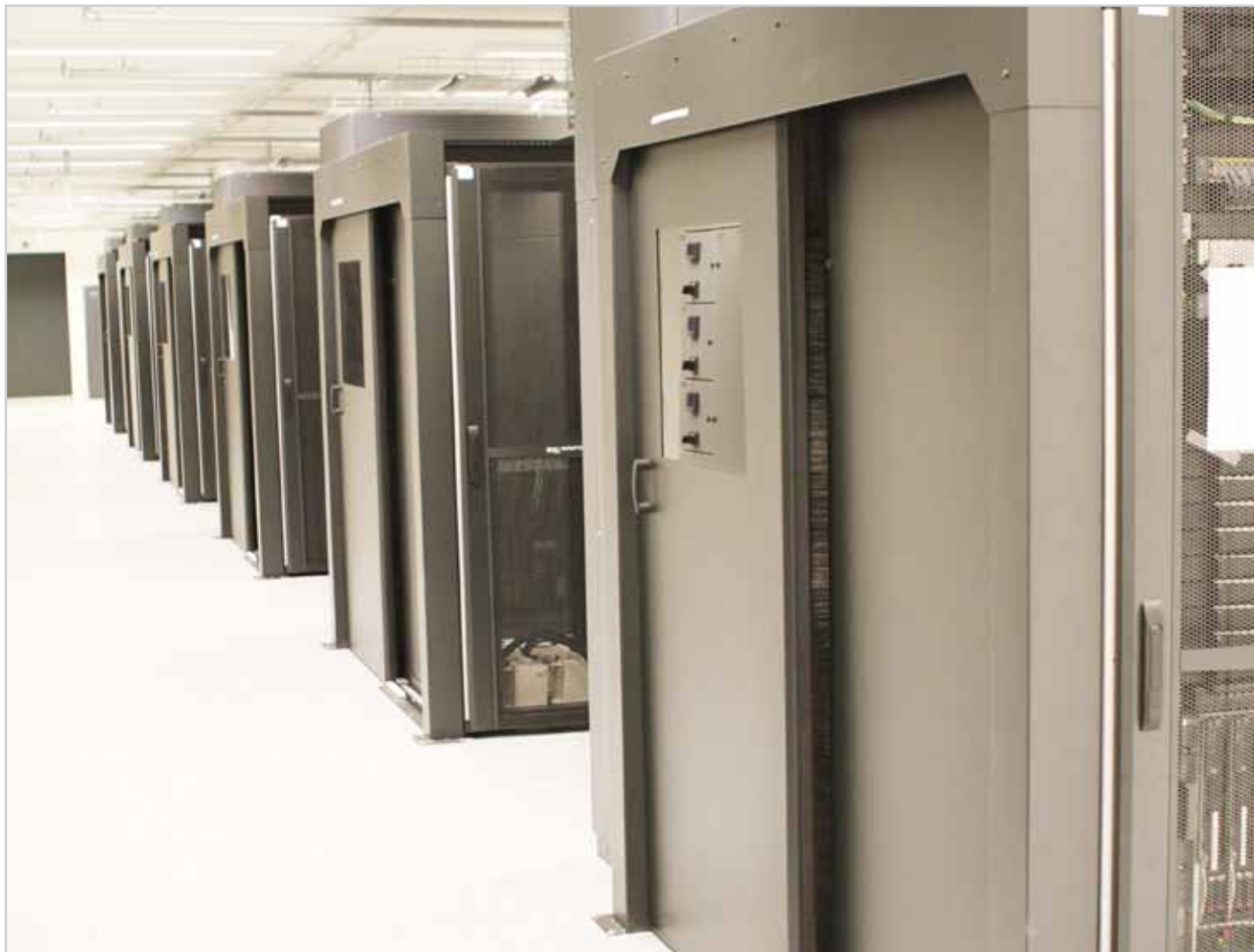
ABB's business partner in Denmark, has delivered a new server room to DONG Energy
