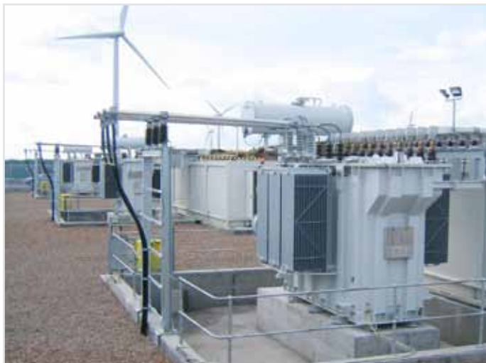
The scope of delivery also included transformers and external water/air heat exchangers
