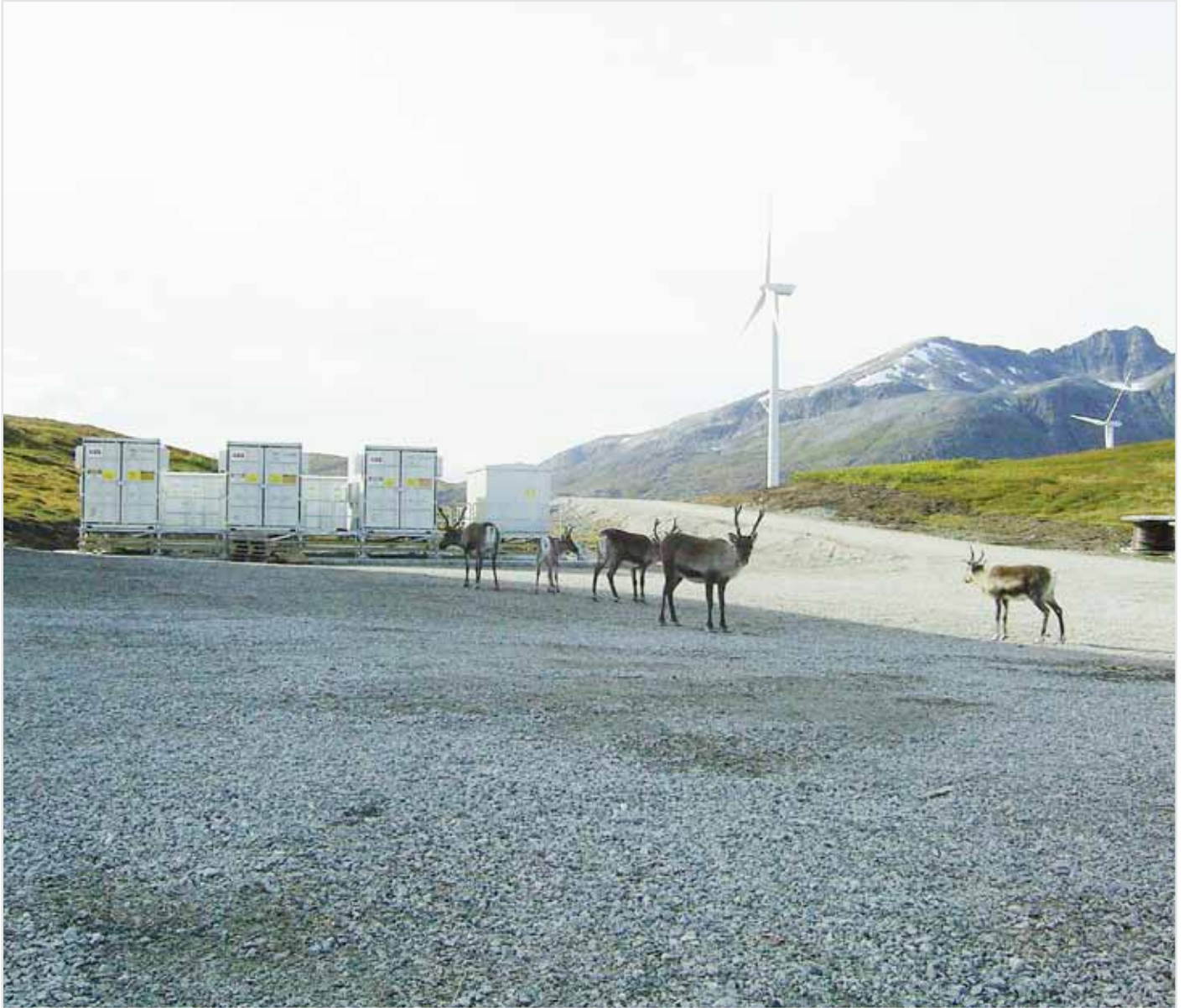
Three 2 MVar PCS100 STATCOM containers for a 54-megawatt onshore wind farm located in Fakken, in the far north of Norway
