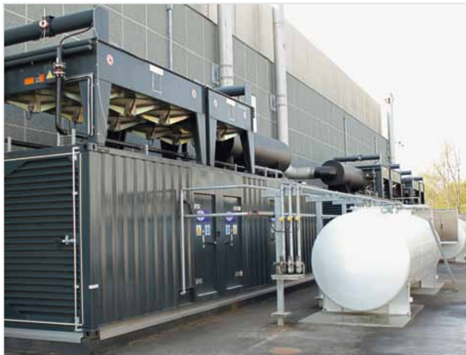
Onsite at DONG Energy's highly energy-efficient data center
