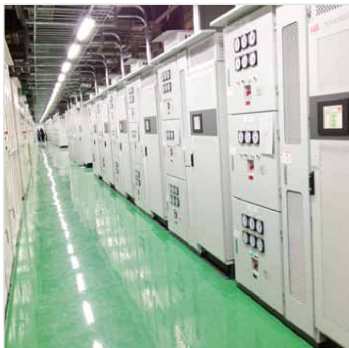
The 32 PCS100 AVCs that are protecting the semiconductor processes
