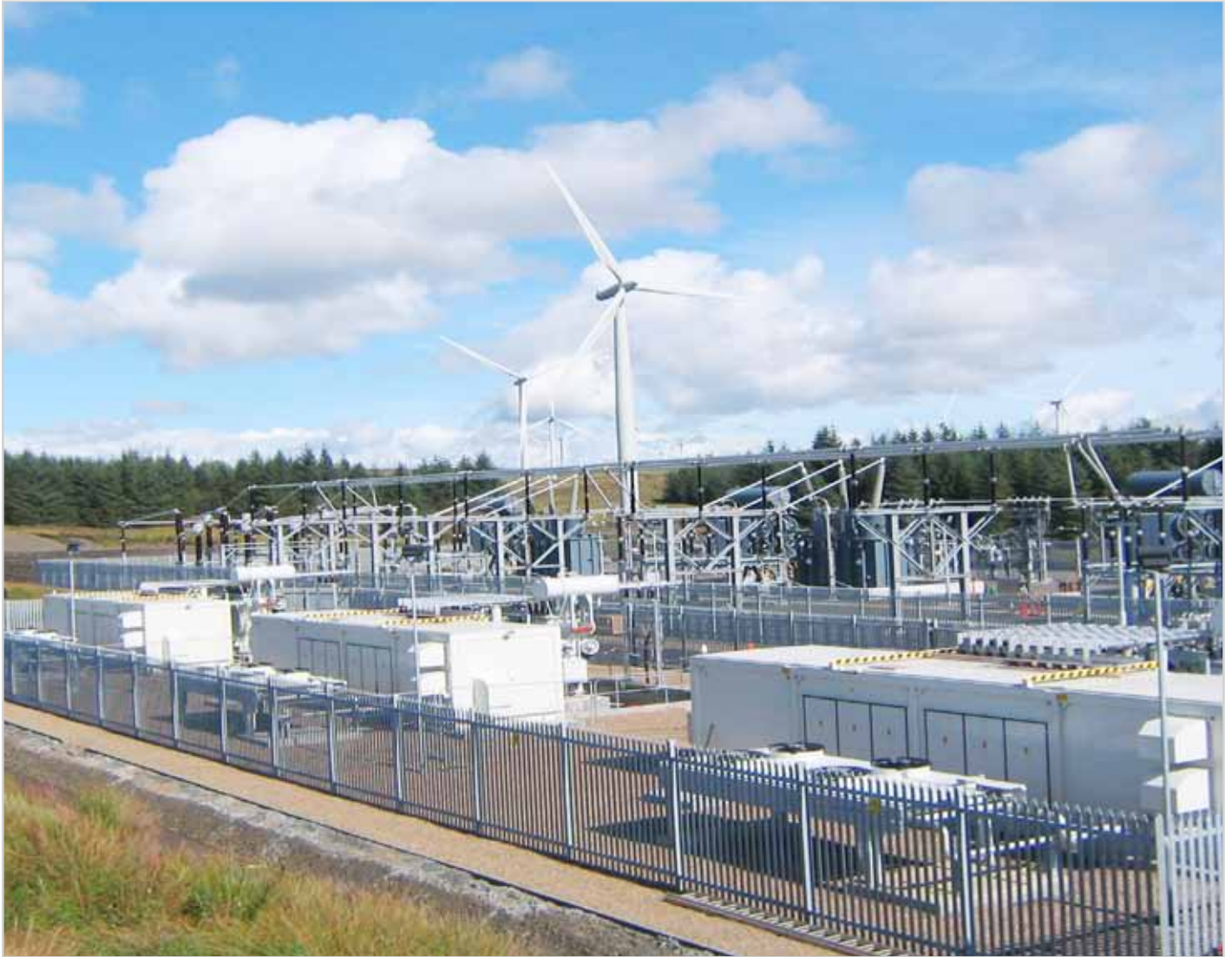
Three liquid cooled PCS 6000 STATCOM units of \pm 15 MVar each at 33 kV installed at Whitelee wind farm, located in Great Britain
