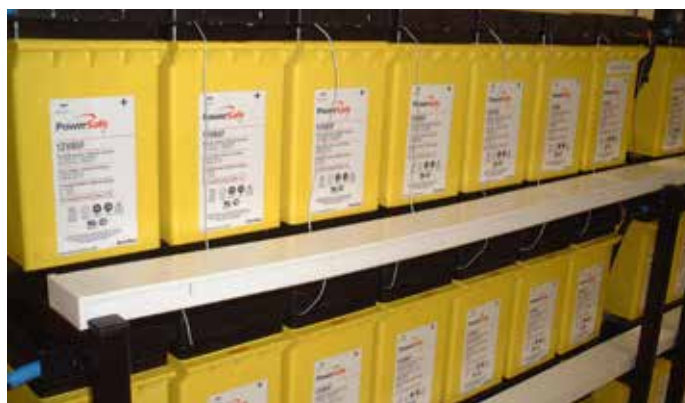
Battery system fitted with AKKA measurement cables.
