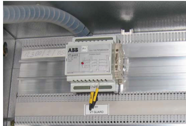
Fig. 5. Connection in the low voltage part of cubicle.
