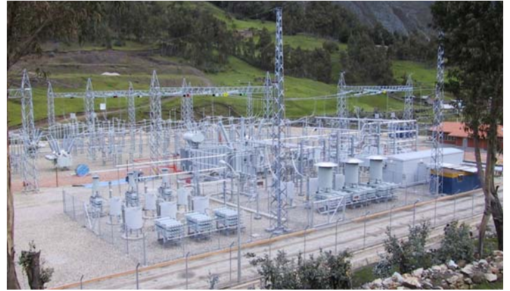
Fig. 10. Site view of the SVC.
