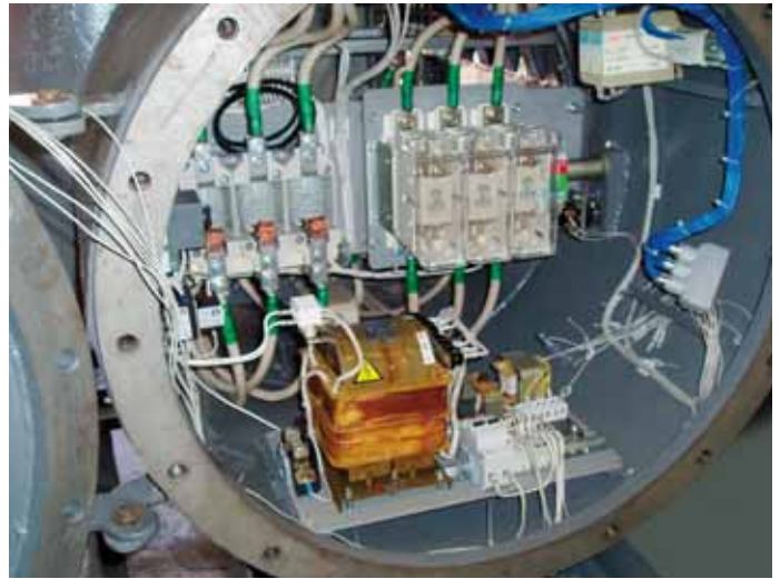
All electrical equipment is protected from the hazardous mine environment to IP54.
