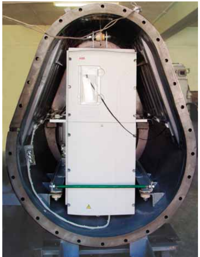
An ABB industrial regenerative drive forms the heart of the rope monorail drive.
