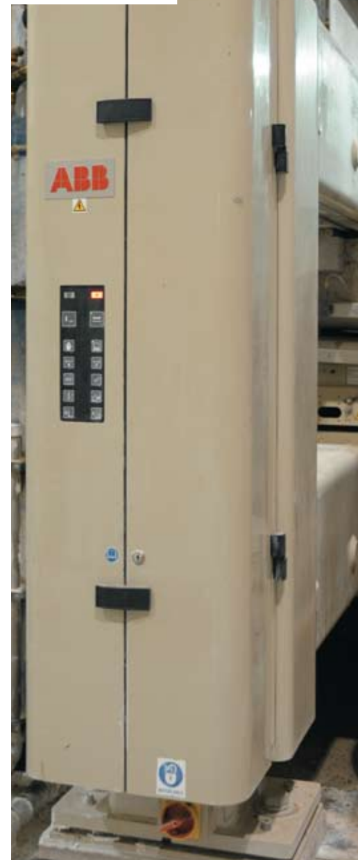
Machine control is accomplished using an ABB 800xA DCS and Smart Platform scanner installed three years ago to replace an aging system.
