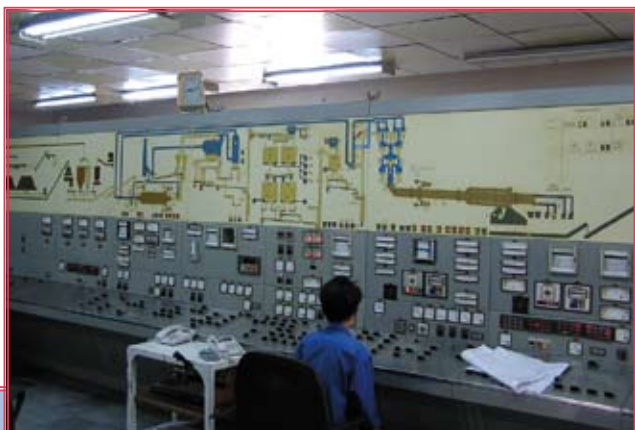
Figure 3. This control room was built in 1964.
