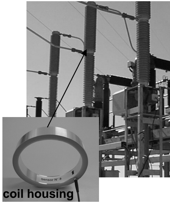
Fig. 1. 170 kV circuit breakers with integrated fiber-optic current transducers.
