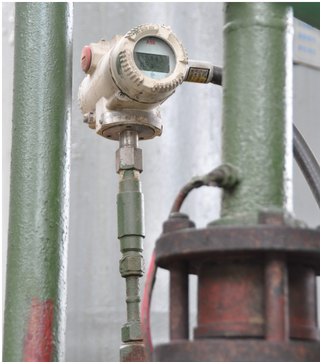
Installed ABB 2600T pressure transmitters
