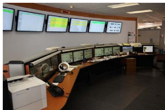
Figure 4 Operator Workstations in IPP
