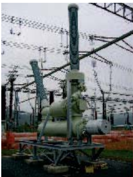
The new 380 kV hybrid switchgear
