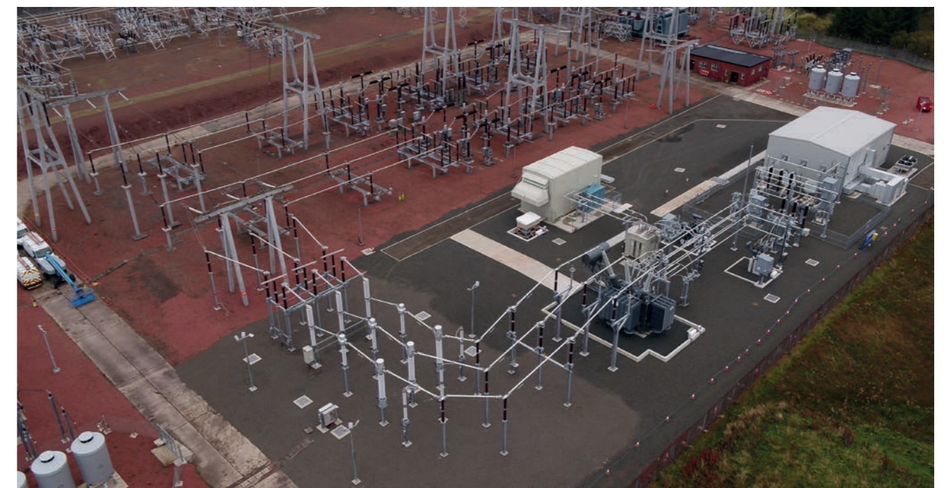
Above: Figure 7. Hybrid synchronous condenser installed at Neilston substation (the Phoenix project)
