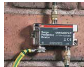
Figure 3. OVR CATV/F mounted in a garage near where the cable enters the building. ... continued overleaf
